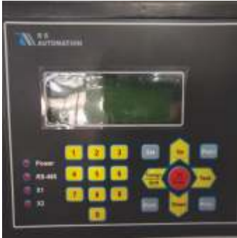
Temperature Data Logger
